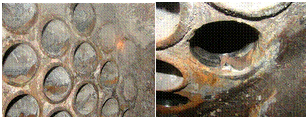
Figure 3. Poorly sealed tubes, biomass boiler, and deformation thereof
