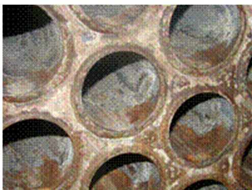
Figure 4. Sediment buildup in a biomass boiler
